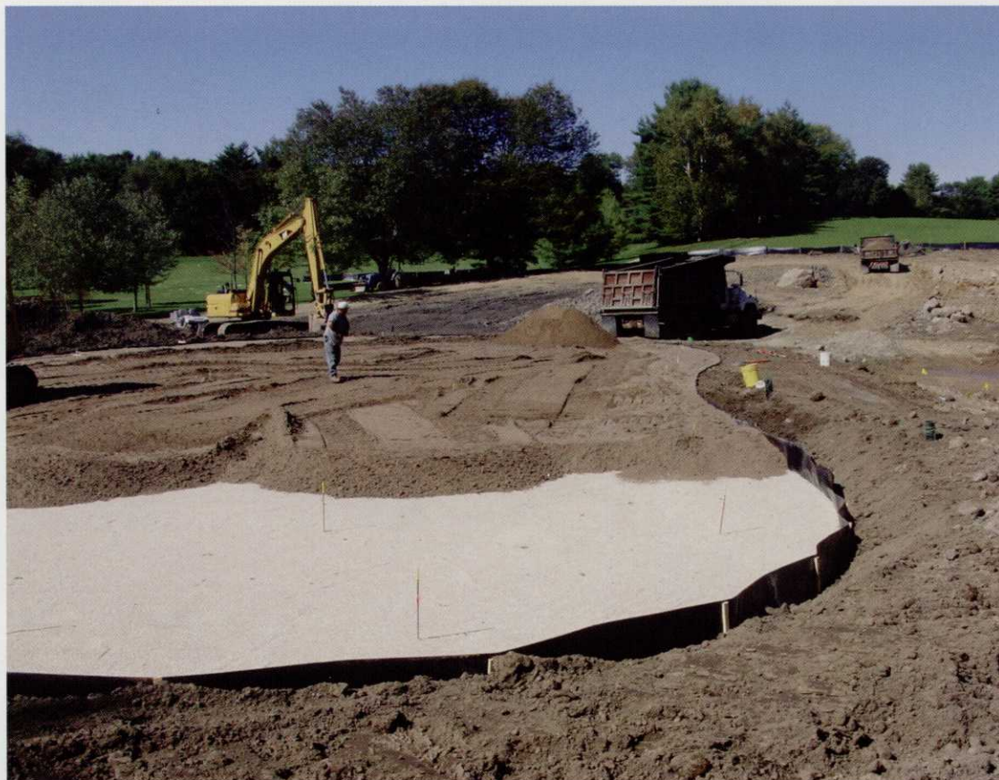
To maximize his maintenance budget, Tony Girardi, CGCS, outsources major construction projects and focuses on daily course maintenance with his staff. Photo: Rockrimmon Country Club
