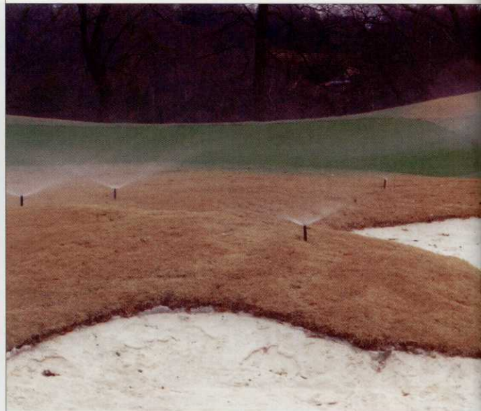
Bunker misters are part of the need to further segregate areas of a golf course that need to be irrigated differently. Photo: Willow Oaks Country Club
