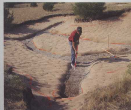
Subsoil makeup and design contribute to the effectiveness of a bunker's drainage. Photo: Professional Turf Products
