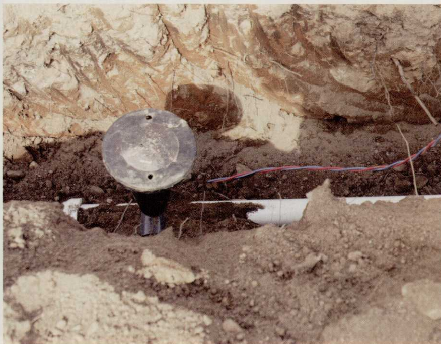
With a decoder system, irrigation can be controlled via the Internet, cell phone or hand-held radio. Photo: EPIC Creative
