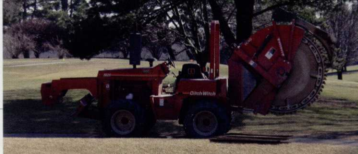
It took the contractor from August 2001 to early June 2002 to install the new irrigation system. Photo: Rockrimmon Country Club
