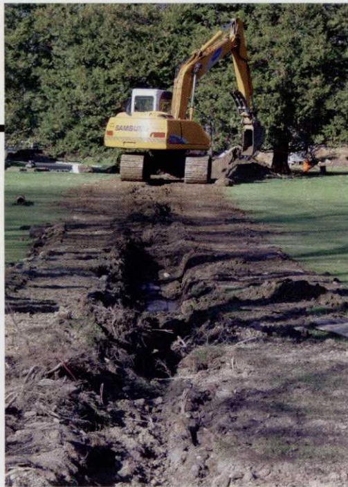
An aging irrigation system caused Rockrimmon Country Club to install a new one. Photo: Rockrimmon Country Club
