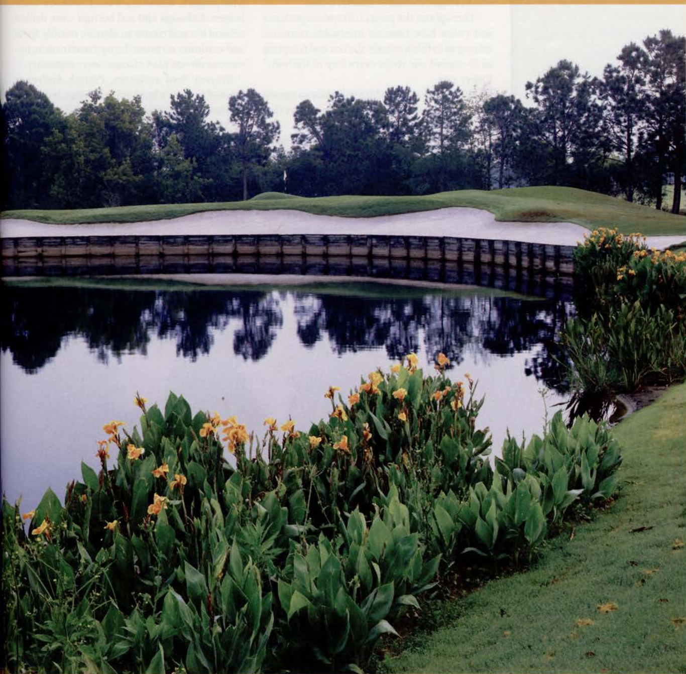
A $3.4-million renovation at Interlachen Country Club included replacing 1,100 feet of bulkhead. Photo: Interlachen Country Club
