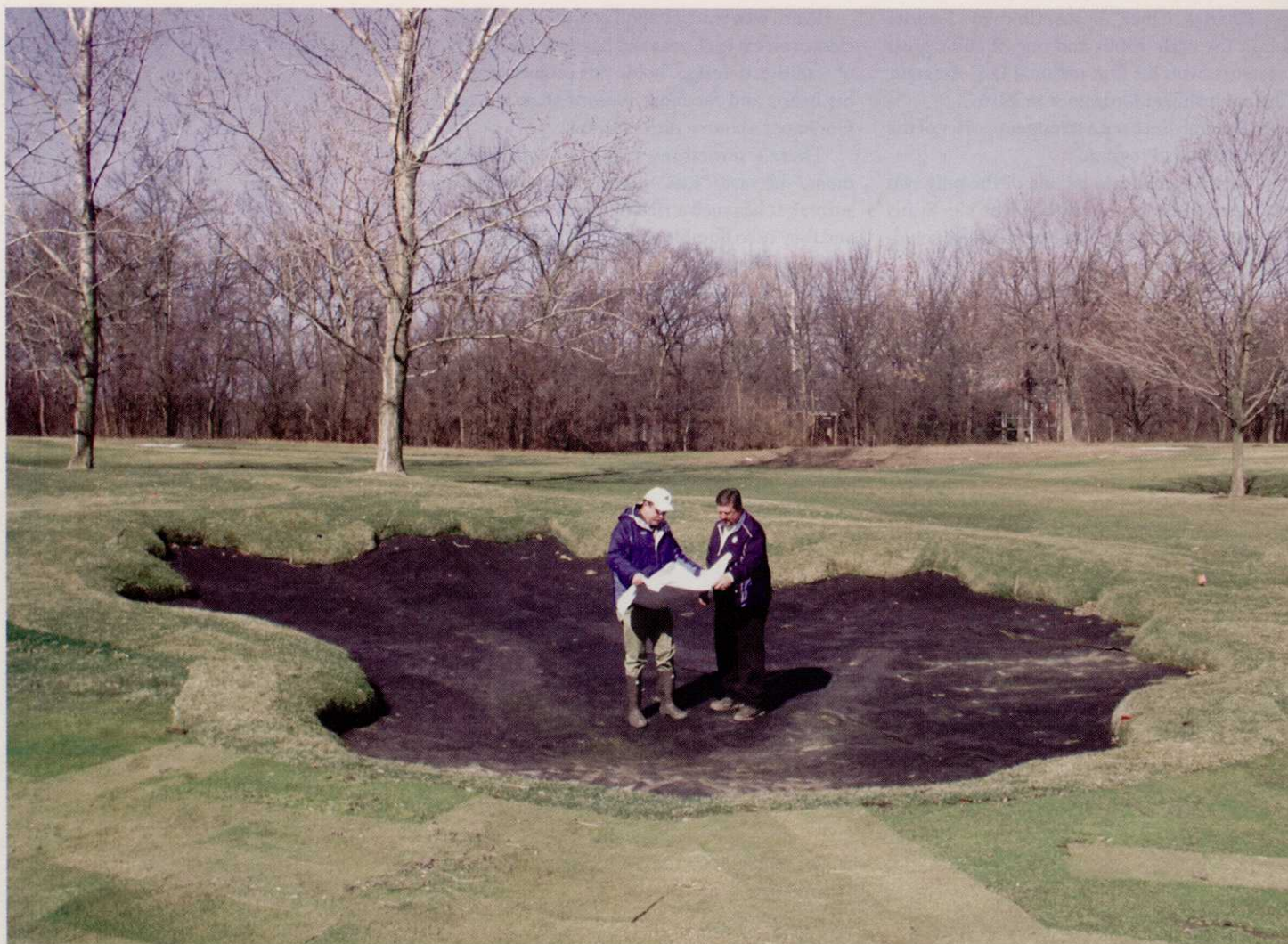
Golf course architect Raymond Hearn and golf course superintendent Robert Lively examine construction plans and a new bunker liner before sand is installed. Photo: Flossmoor Country Club
