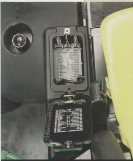
John Deere's White Box determines where power interruption occurs. Photo: John Deere
