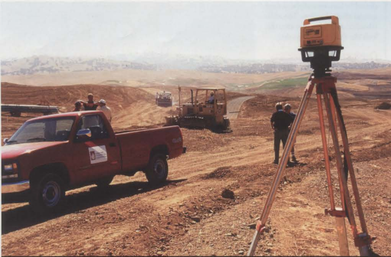
Centralized decision-making, in combination with a set project budget and scope, speeds decision-making in design-build projects, and reduces change orders.
