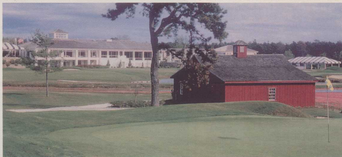
In building nine new holes at Willowbend Golf Club in Mashpee, Mass., ASL had to line fairways and tees and greens surrounds with rubber to protect the site's environmental and historical lands.
