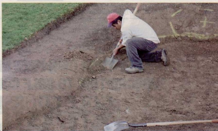
A worker excavates a bunker to bring back the fat lip of Fazio's original design.
