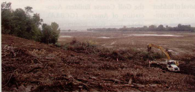
Work continues at the Jewel, which is scheduled to open in July 2004.
