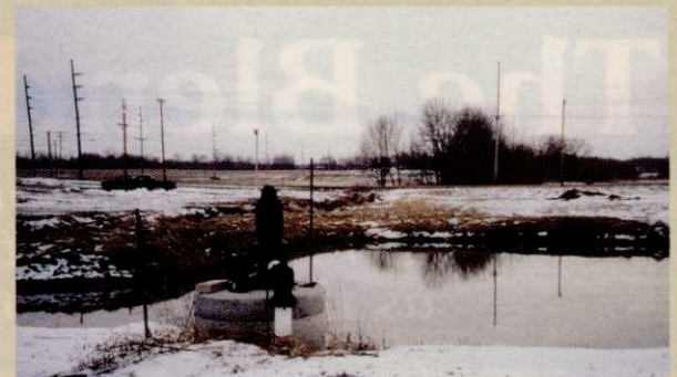
Effluent is pumped into a lagoon before being piped to the course.
