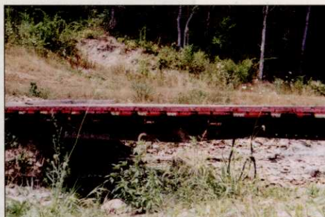
The bridges at Buck's Point GC were constructed from the decks of old tractor-trailers.
