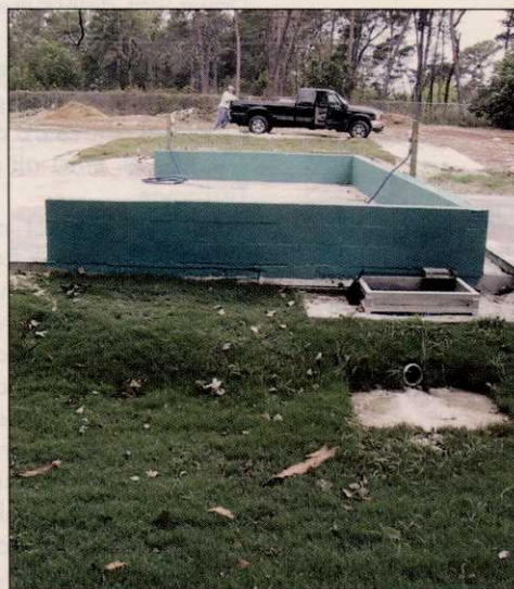
An installed SurfRax system at Miles Grant CC
