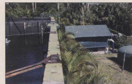
A storage tank keeps a ready supply of effluent.
