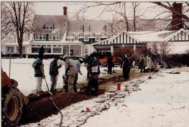
Winter projects, such as this irrigation project at Oakmont CC, in Pennsylvania, have been frustrated by harsh weather in the Northeast.
