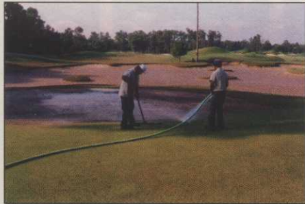
Hoses and squeegees were required to remove layers of silt from greens at the Northgate CC.
