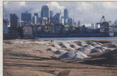
View of construction on Serapong's 14th hole, with harbor and skyline in background
