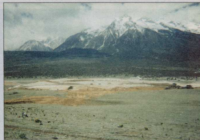
Holes 10, 11 and an irrigation lake, fed by underground glacier rivers, under construction at Nelson and Haworth's Jade Dragon Snow Mountain Golf Course in China.
