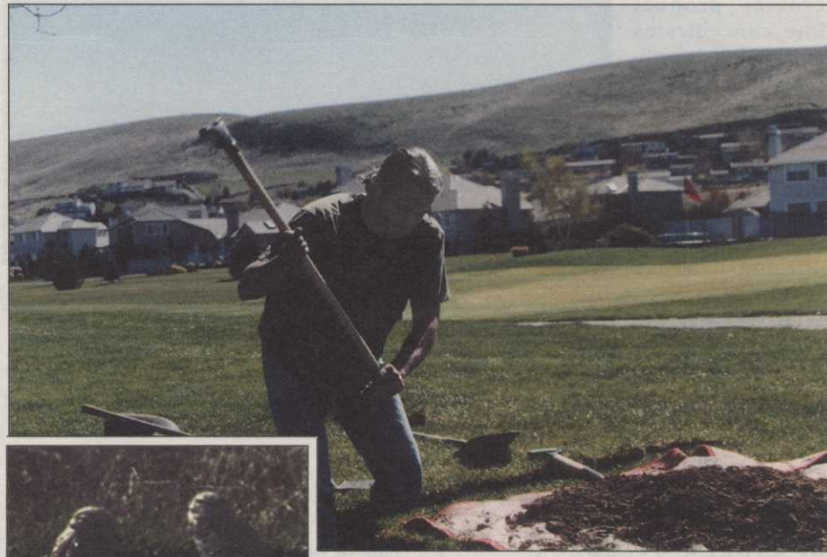
Project Coordinator Matthew D. Smith digs a trench for an artificial owl burrow that is situated just 33 feet from the 16th green at Canyon Lakes Golf Club in Kennewick, Wash. (above). A pair of burrowing owls (inset).
