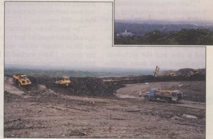
It took an average of 800 trucks a day for three years to bring 7.7 million cubic yards of fill from the Big Dig to Quarry Hills. A view of the Boston skyline from the site. (inset)
