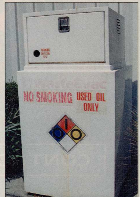
Used oil is pumped into an outside container and then hauled away.
