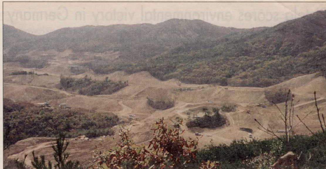
A typical Korean golf course construction scene: Nickels' Mauna Ocean Resort course slowly takes shape along the hillsides.
