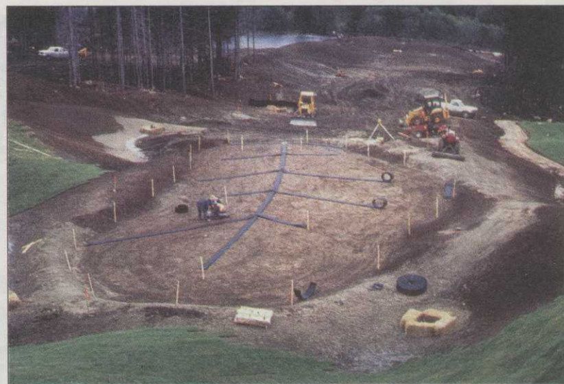
One of the earlier Hurdzan-Fry flat pipe installations. See GCN March, page 45.
