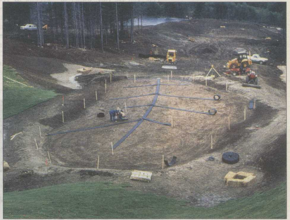
One of the earlier Hurdzan-Fry greens showing ADS AdvanEDGE pipe installed horizontally on the sub-base.
