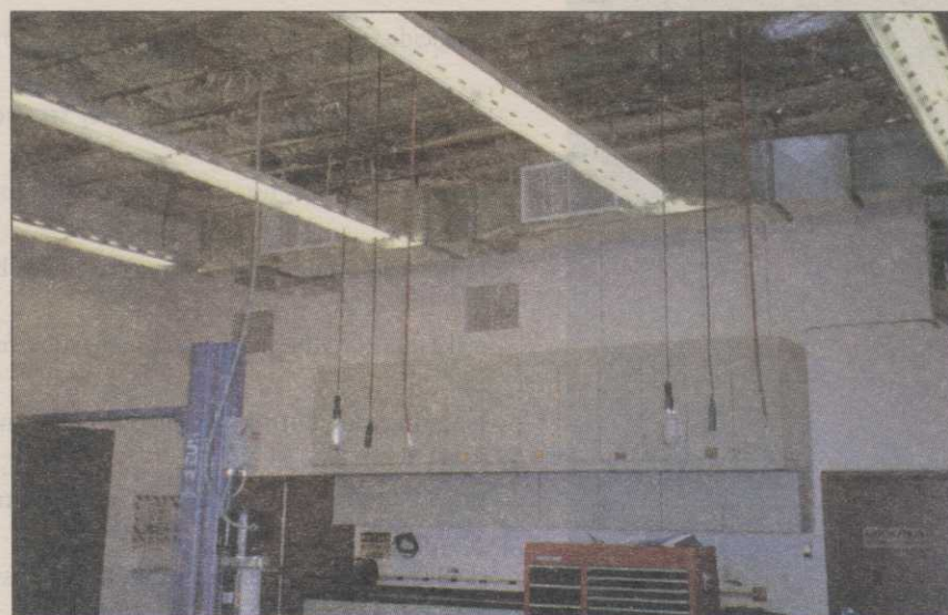
The modern maintenance shop can have many accessories that are mounted overhead for easy access.
