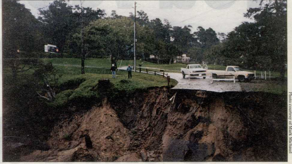
Access to the 15th tee at Pebble Beach Golf Links is destroyed as a result of the El Niño-driven storms in early February.
