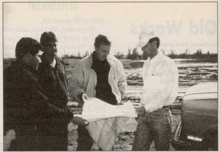
Hale Irwin, second from right, looks over the site for the new Grand Southern Golf Course, under construction in Tunica, Miss. With Irwin are, from left, Bryce Swanson of Hale Irwin Golf Services, Russell Durbin of Landscapes Unlimited (the builder), and Stan Gentry of Irwin Golf Services.
