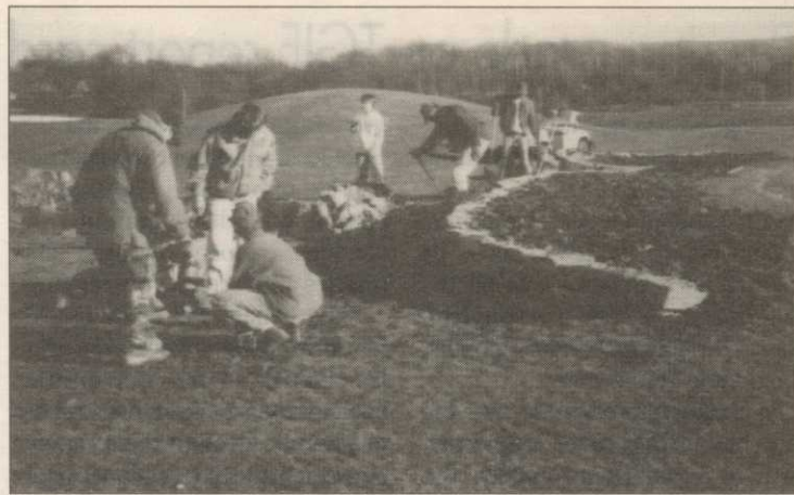
Students build a retaining wall at one of 10 sites on Penn State's newly redesigned Blue Course.
