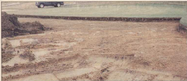
The 14th green shows the old root-zone material (left) that was removed by Tectonic, Inc. and grounds maintenance crews at Keystone Ranch golf course. The front of the green was left open for play during reconstruction. Note the heavy organic material in the soil profile, along with the deep-core aerification holes that were back-filled with sand.
