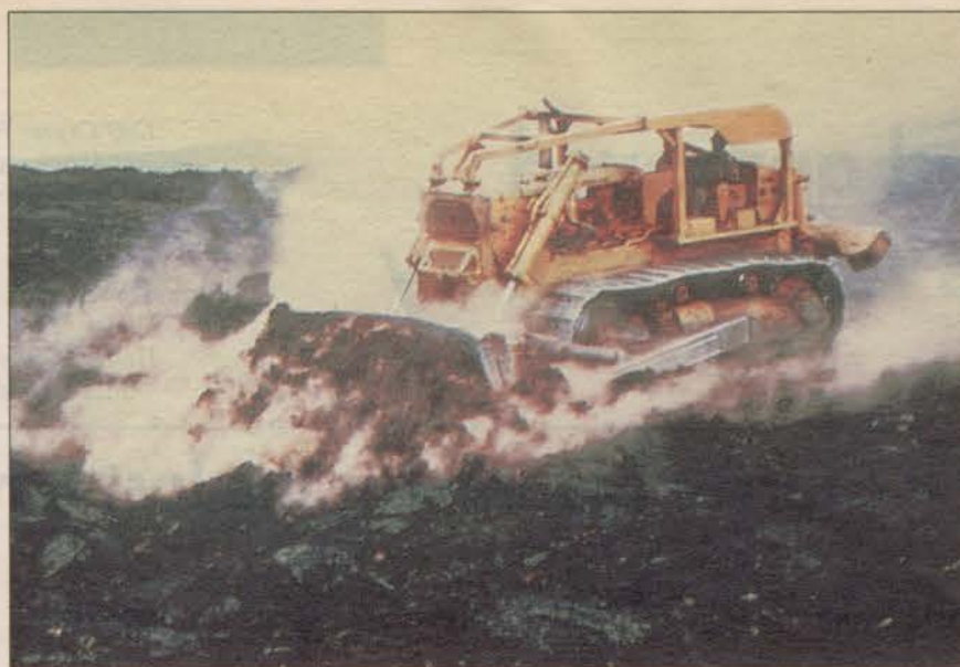
A bulldozer crushes lava as it tracks over a site in Hawaii. The work is a balancing act between heavy-duty rock-moving and taking care not to destroy an area the architect wants to incorporate into his design.
