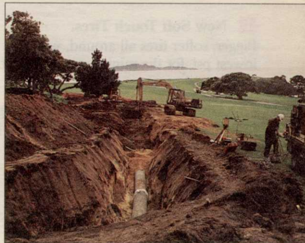
Effluent pipe is laid along the 14th fairway at Pebble Beach Golf Links.
