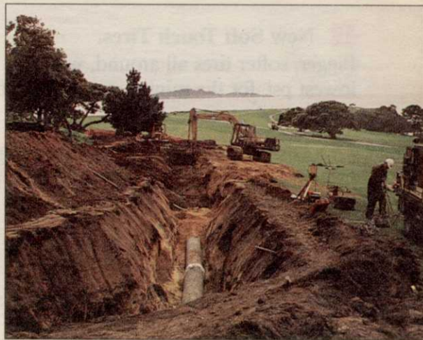
Effluent pipe is laid along the 14th fairway at Pebble Beach Golf Links.
