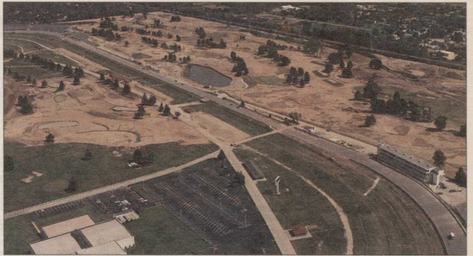
The newly renovated Speedway course will feature 18 holes — down from 27 — with four inside the oval.
