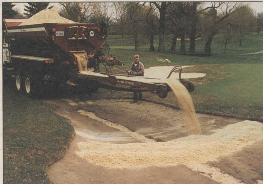
After the bunkers at Scioto Country Club were totally renovated, The Placer installed sand at an initial six-inch depth on the bottoms and two to three inches on the slopes with minimal handwork.
