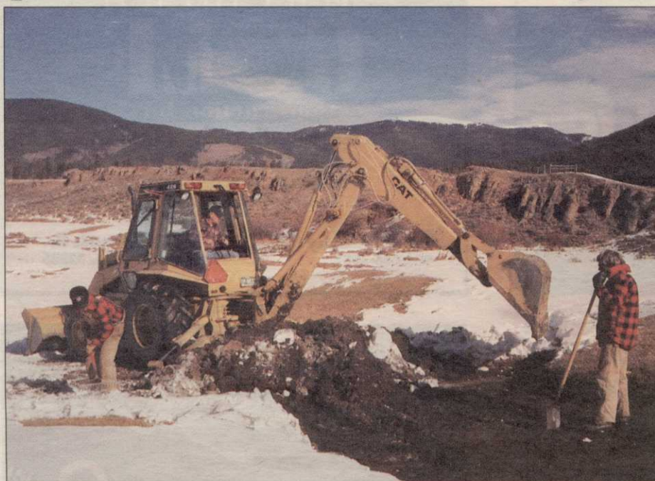
Two Keystone Resort maintenance crew members help a Tectonic backhoe operator clean out a bunker.
