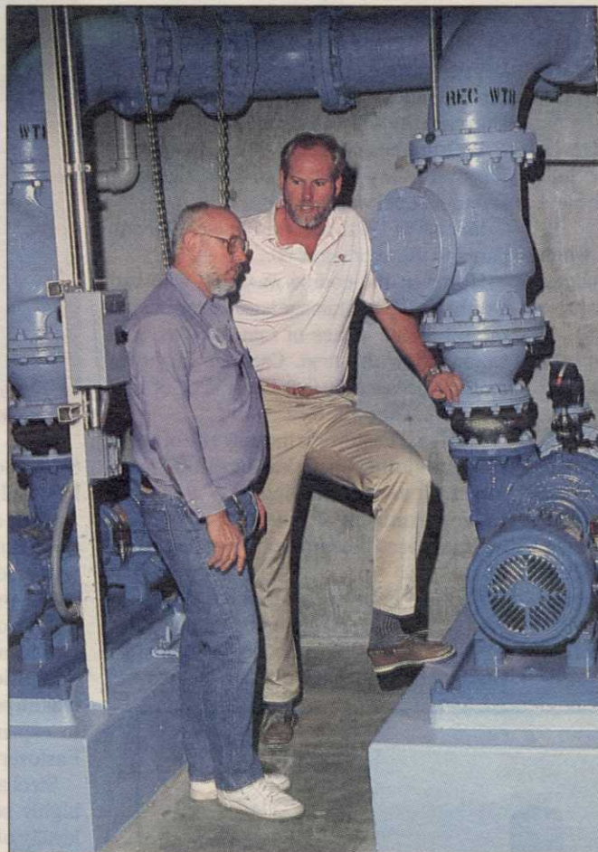
George Corthouts, rear, discusses water treatment with Jim Tombaugh, treatment plant manager, inside the plant.
