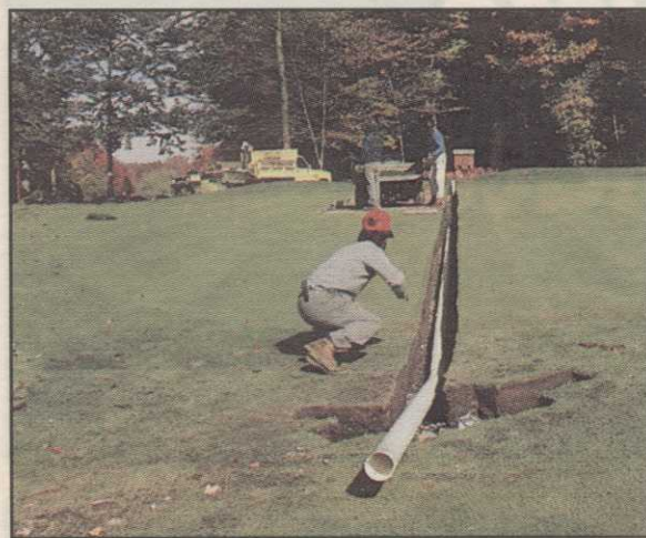
Workers at Burning Tree CC install PVC pipe to solve a drainage problem on the 15th green. They first had to drill through the putting surface and underlying ledge with a jackhammer. Superintendent Steve Renzetti reports the 15th is now one of the top greens on the Greenwich, Conn., layout.
