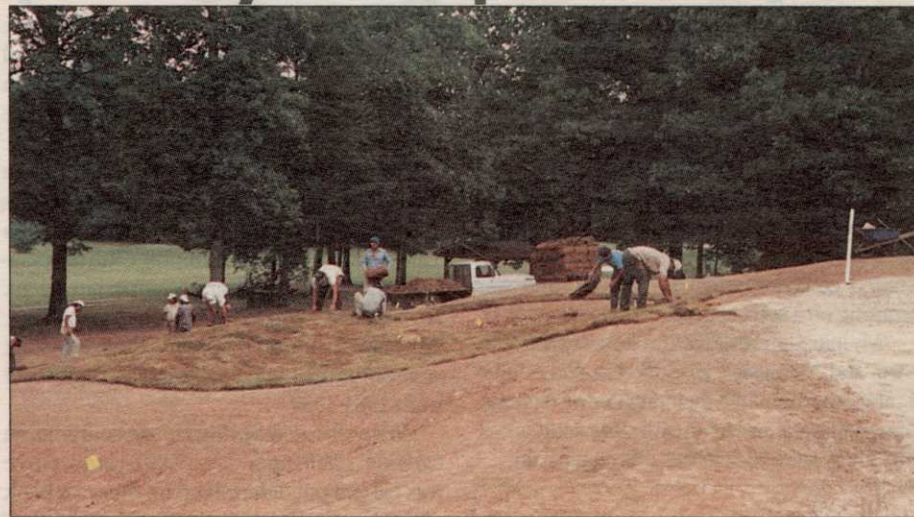
A crew from Chantilly Turf Farms, Inc. lays bluegrass sod on the perimeter of the 13th green at International Town and Country Club. Chantilly, a subcontractor to John Ponko Inc., will put down bentgrass sod on the greens. Chantilly grew the bluegrass sod, while Summit Hall Turf Farm grew the bentgrass.
