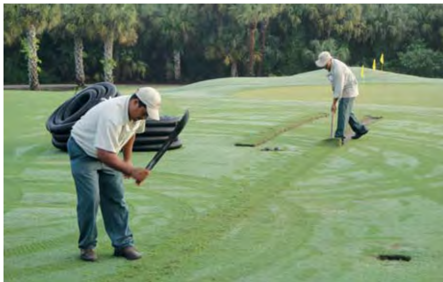
Use a 12-inch wide sod cutter blade to make the initial cut on the painted drain lines. Photo by Darren Davis.
