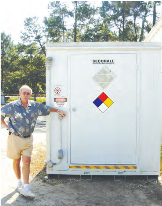
Superintendent Doug Abbuhl stands next to the new self-contained chemical storage building by the old maintenance building. Photo by Joel Jackson
