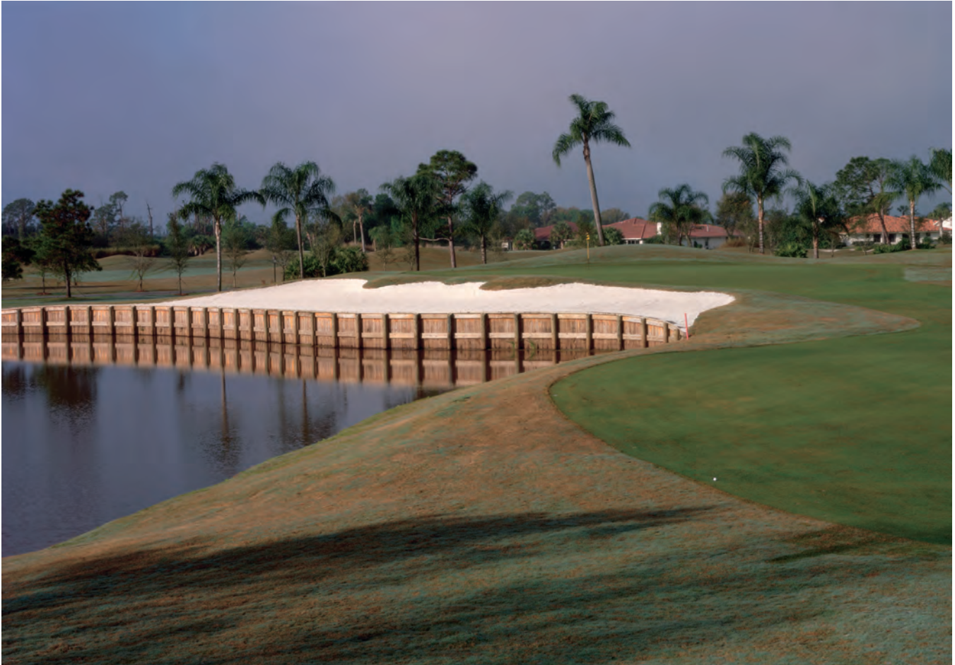
The new bulkhead on No. 6 is evidence of the five acre expansion in lake area to generate fill for the new mounding and to store more irrigation water. Photo by Daniel Zelazek.
