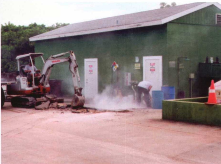
Demolition of the old slab outside the chemical room. Note containment around the fertigation tanks to the right.
