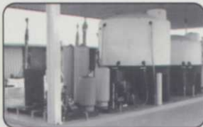
Wash Rack Systems – •closed loop •sewer discharge
