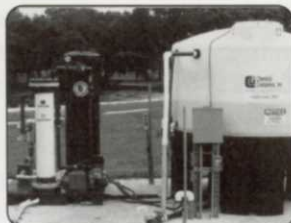
Sewer Discharge System
