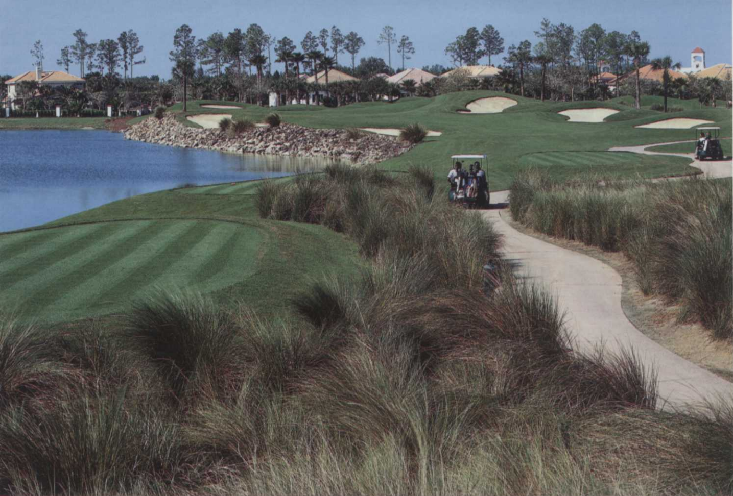
Limestone bedrock excavated during construction is used on several holes, shown here on #8, to stabilize steep lake banks and provide interesting texture contrasts. Photo by Daniel Zelazek
