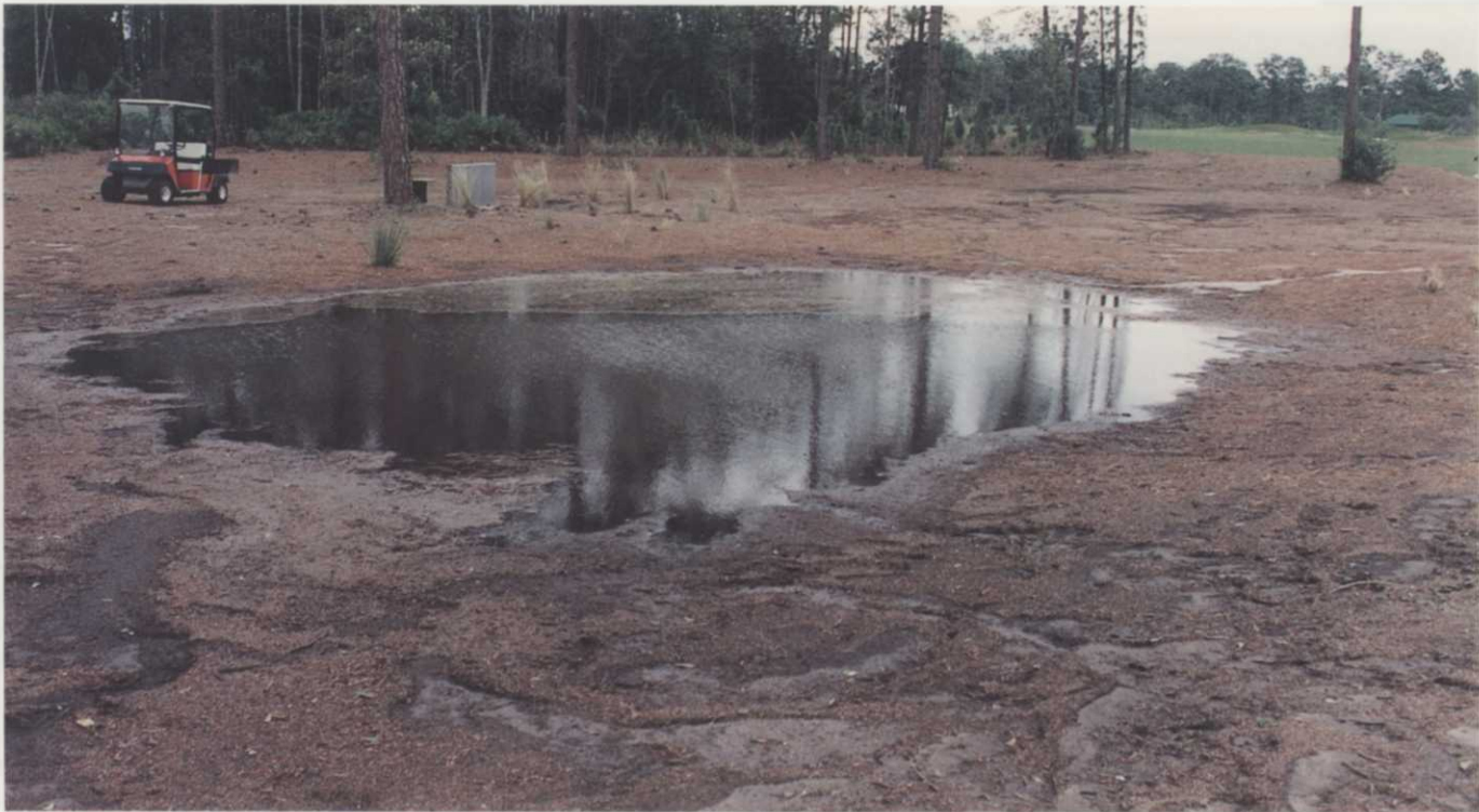
A clogged drain basin produces an unexpected water hazard. Superintendents have been known to take off their shoes and roll up their pant legs and wade in to solve the problem temporarily. Eventually the sloping pine straw areas are sodded, and work turns to more important jobs, like grooming the turf. Photo by Joel Jackson.
