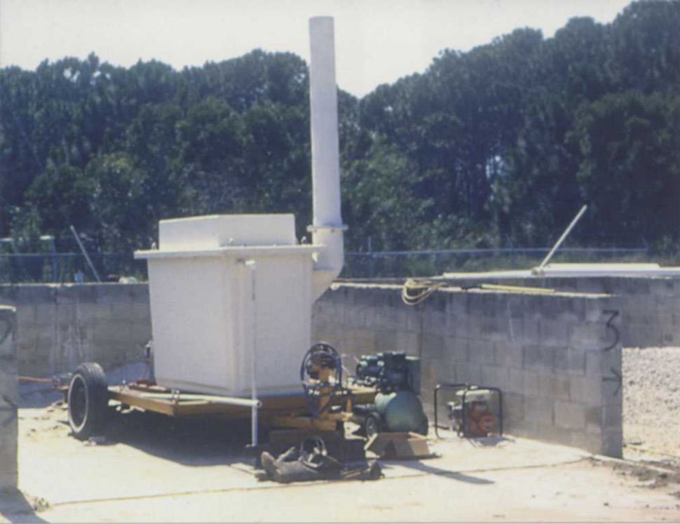
Contaminated groundwater requires special equipment like this stripping tower to remove residual material.
